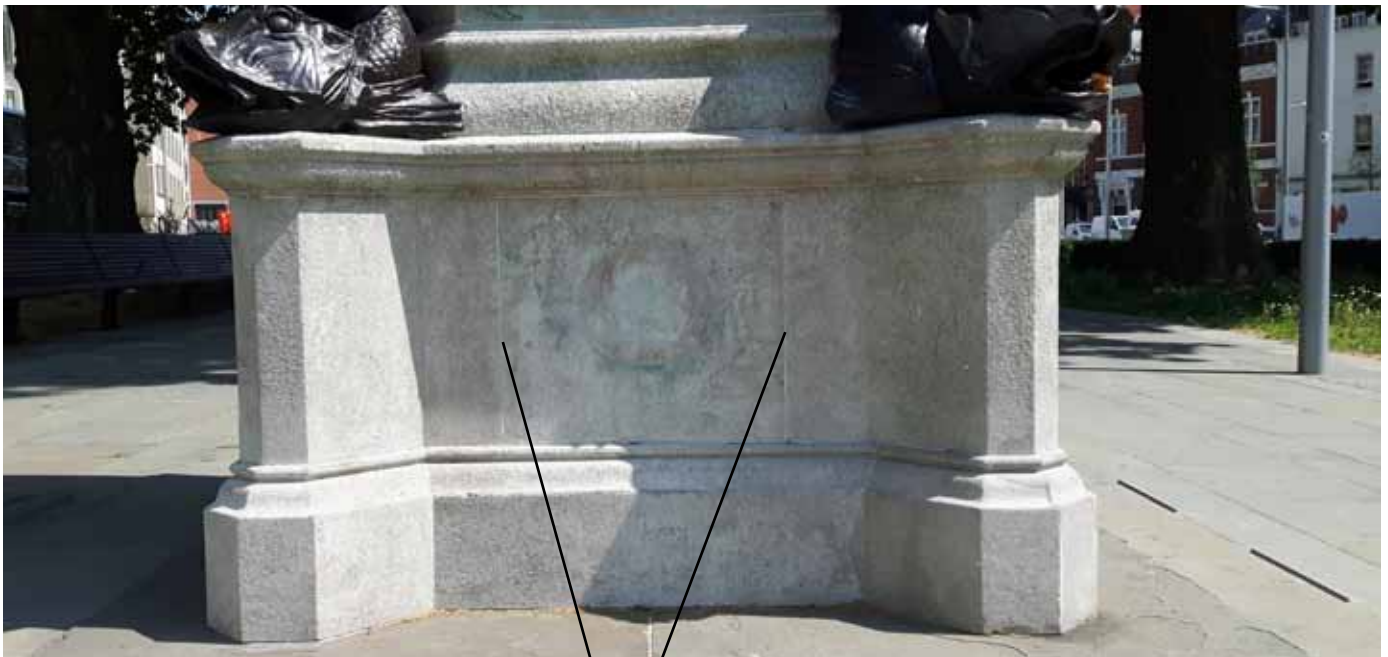
Mortar joints on pedestal
